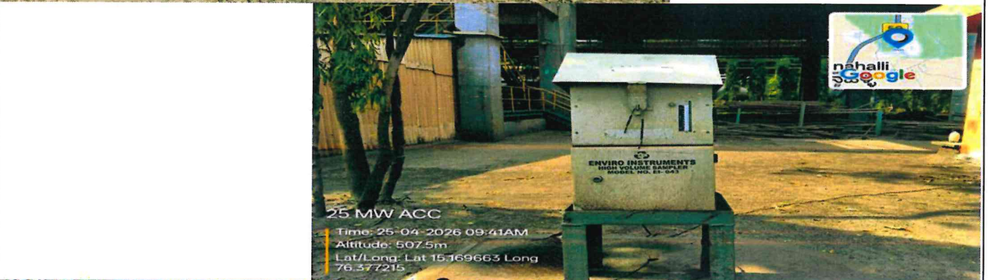
25 MW ESP Time: 24-04-2026 10:19AM Altitude: 459.1m Lat/Long: Lat 15.170421 Long 76.377571
